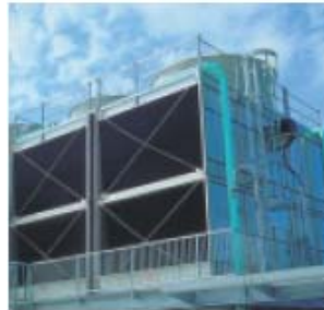
Figure 38: Large cooling tower.
