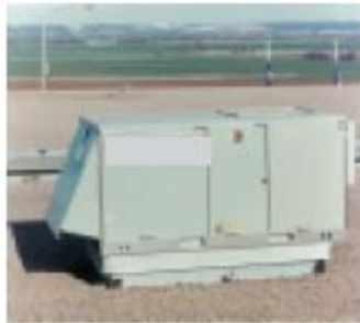
Figure 11: Small rooftop air handling unit.
