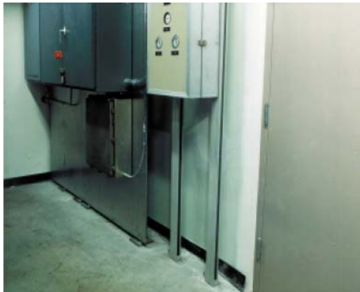
Figure 156: Two different ways to support control panels: using a metal plate attached to floor and ceiling with steel angles (left); using struts extending to floor and ceiling (right).
