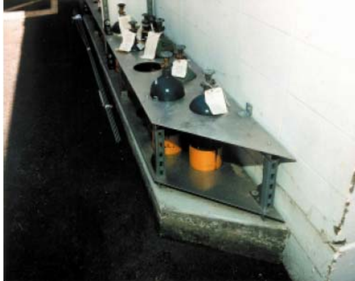
Figure 81: Small gas cylinder storage.
